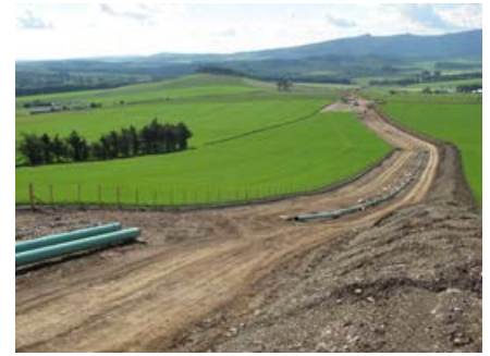
Part of the Moray Reinforcement High Pressure Gas Pipeline route during construction.
