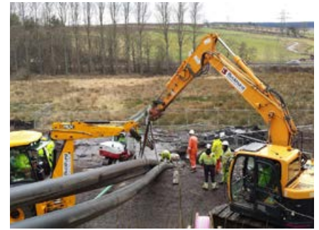
Part of the Blackhillock to Keith 275kV Underground Cables route during construction.
